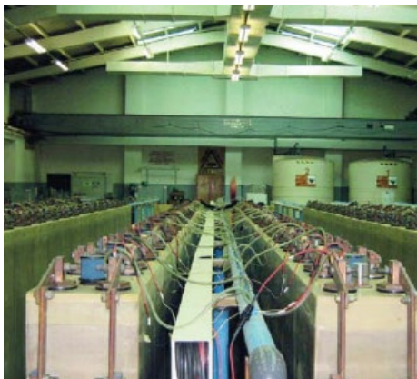
Battery Charging Hall
