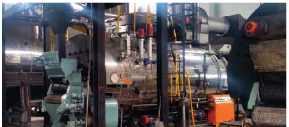
Boiler Electrical Installations
