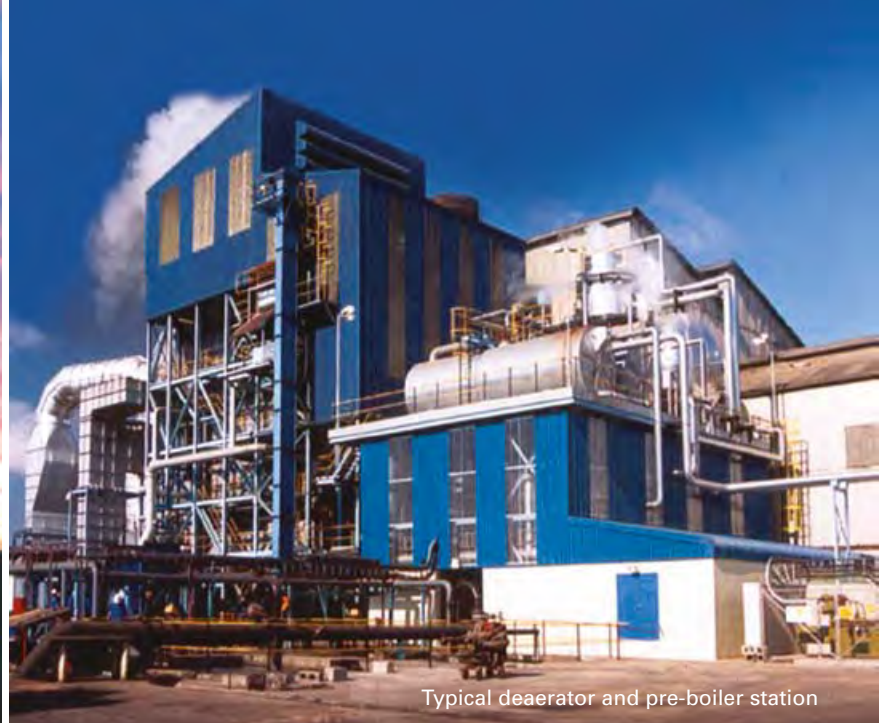
Typical oil refinery boiler
