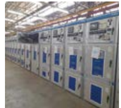
Medium Voltage Panel
