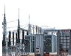
Power Transformers Station
