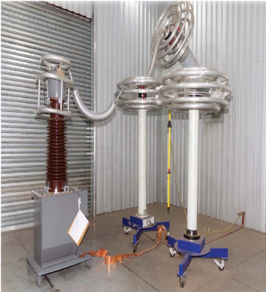
132kV CT's during electrical testing
