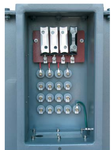
LV terminal enclosure is of a weatherproof type and fitted with a sliding cover
