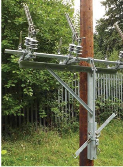
Single Pole Mounted unit
