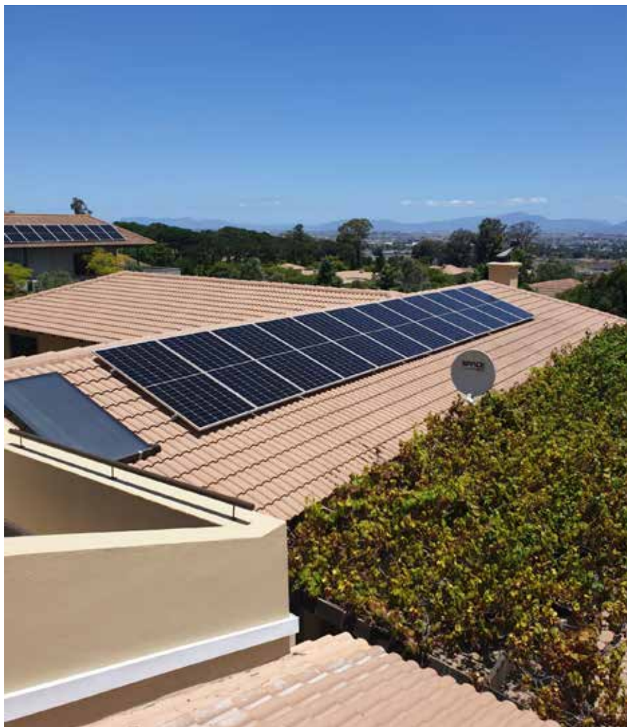
One of Satchwell's residential PV solar systems that have been supplied and installed around the country since its introduction into the market late last year.
