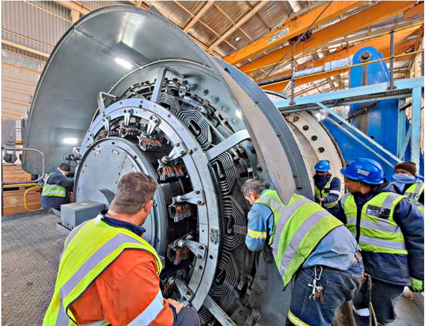
Danie Gouws, M&C's Chief Field Service Technician, (in orange shirt) assists the mine's technical personnel in the installation of the rock-winder motor into the man-winder position.
