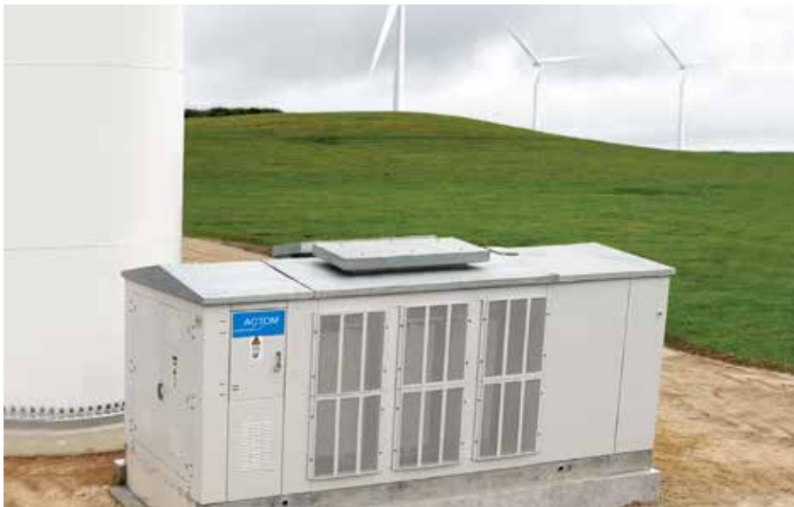
A 2.8MVA pad mounted transformer kiosk (PTK) in use at the Golden Valley Wind Farm near Cookhouse in the Eastern Cape.
