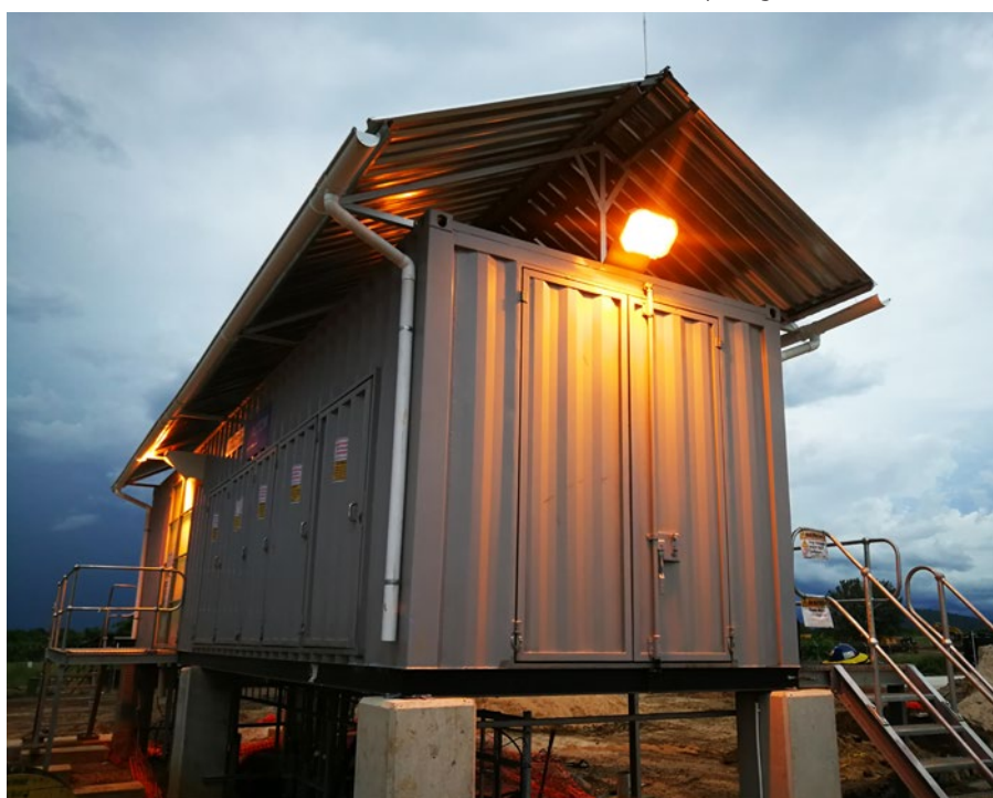
A prefabricated collector E-house substation, equipped with medium voltage switchgear for solar.
