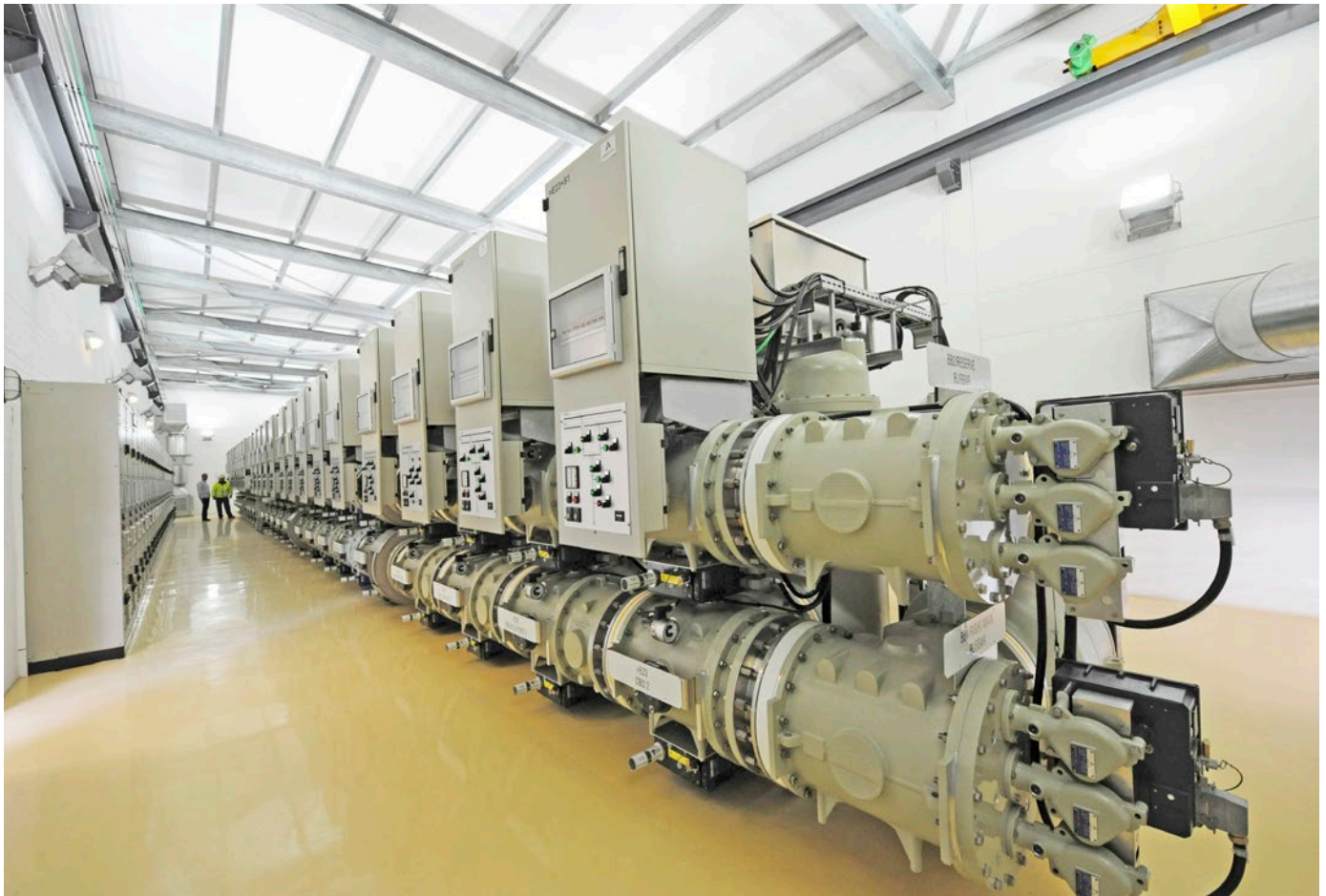
A view of the GIS switchgear in the City of Cape Town's 132kV Foreshore indoor substation, for which Power Systems supplied and installed the electrical works in 2009.
