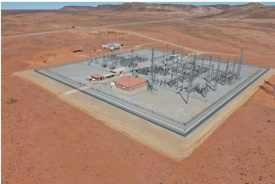
The Groeipunt substation between Springbok and Aggenys in the Northern Cape connects the Kangnas wind farm to the grid via ACTOM's 250MVA 220/132/22kV transformer and related substation equipment.
