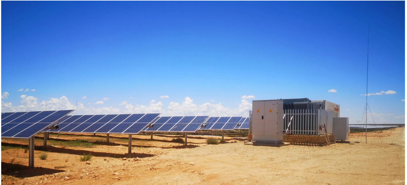
ACTOM Distribution Transformers supplied this 2750kVA 33kV/690V Dyn5 Pad-Mount Transformer Kiosk (PTK) installed at Greefspan 2 Solar Park in Douglas, Northern Cape.
