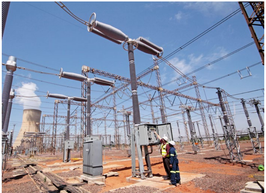
High Voltage Equipment's Craig Aaron and Service Technician Mpho Makgae check the spring operating mechanism for the first of five 550kV replacement circuit breakers installed at Duvha power station.
