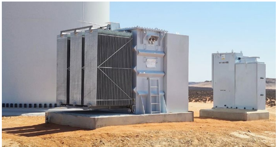
A 2.7MVA 690V to 33kV step-up pad mount transformer is installed at the Kangana Wind Farm in the Northern Cape.
