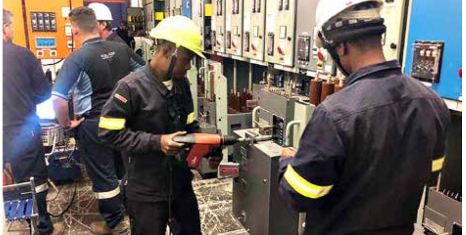
Technicians of MV Switchgear and WPI Power Solutions' Rustenburg Branch conduct routine maintenance work on an electrical installation at one of the mines served by the branch.
