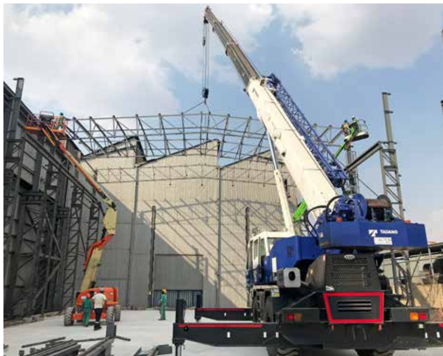
The UBE unit's large mobile crane is shown in action at a construction site.
