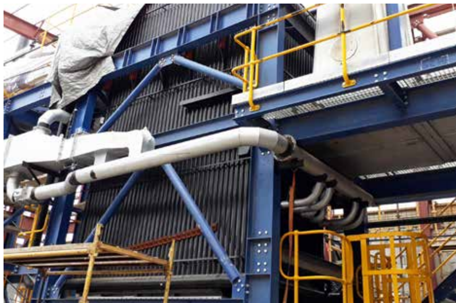
The installation of a Torripac boiler in Grenada - shown here is the vibrating grid.
