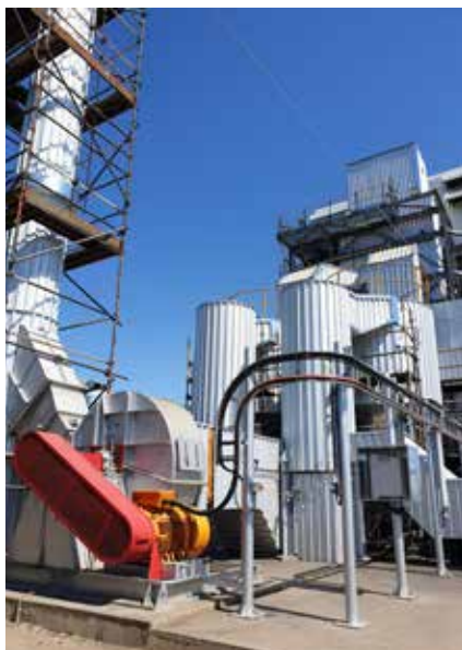
A MicroGen installation in Ladysmith, KwaZulu-Natal.
