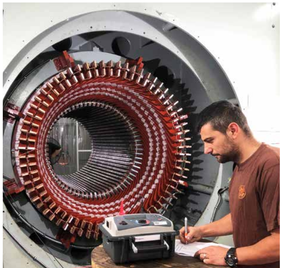
Test Technician Sergio Bernades conducts tests on a 36MW stator rewind at M&C Power Generation.
