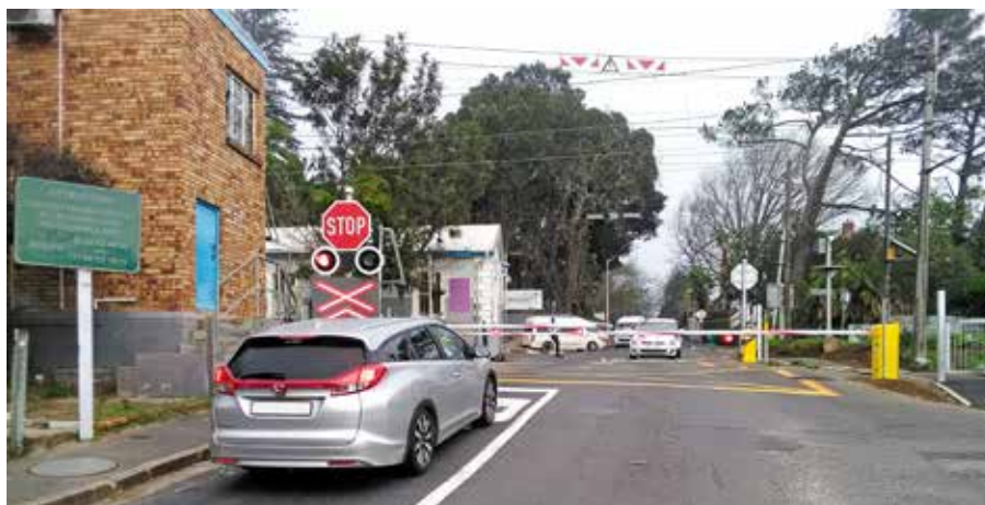
A view of Kenilworth Road showing the new half-arm booms that have been installed to control traffic at the level crossing.
