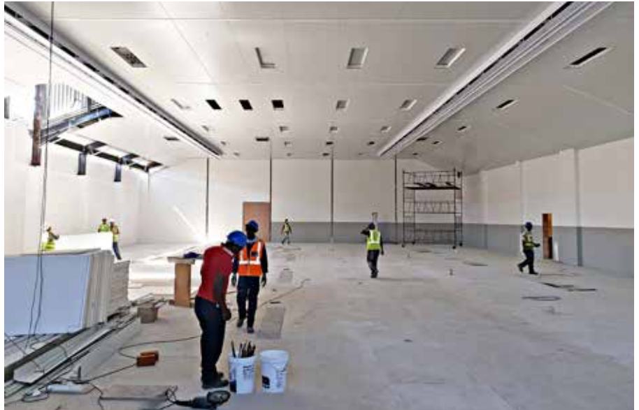
The rebuilding of the weaving shed at Colibri Towelling's Strand plant nears completion.
