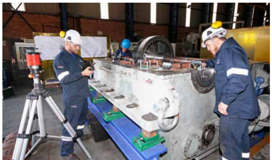
Raymond Saayman, a Turbine Fitter; Zondwane Moleboheng, an Apprentice and Anthony Mancera, an Assistant Turbine Fitter using the latest laser levelling and alignment tool.
