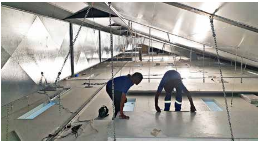
The LED lighting will be installed from the top in the rectangular openings as shown in the walkable ceiling, while the central vacuum system and compressed air will also be installed above the ceiling for connection to the weaving machines below – all to allow easy maintenance.
