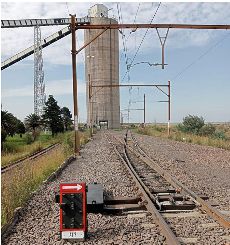
One of three point sets with indicator that form part of the semi-automated yard control system ACTOM Signalling installed recently on the line serving ATC's Impunzi mine's loadout station. The coal silo above the loadout station is seen in the background.
