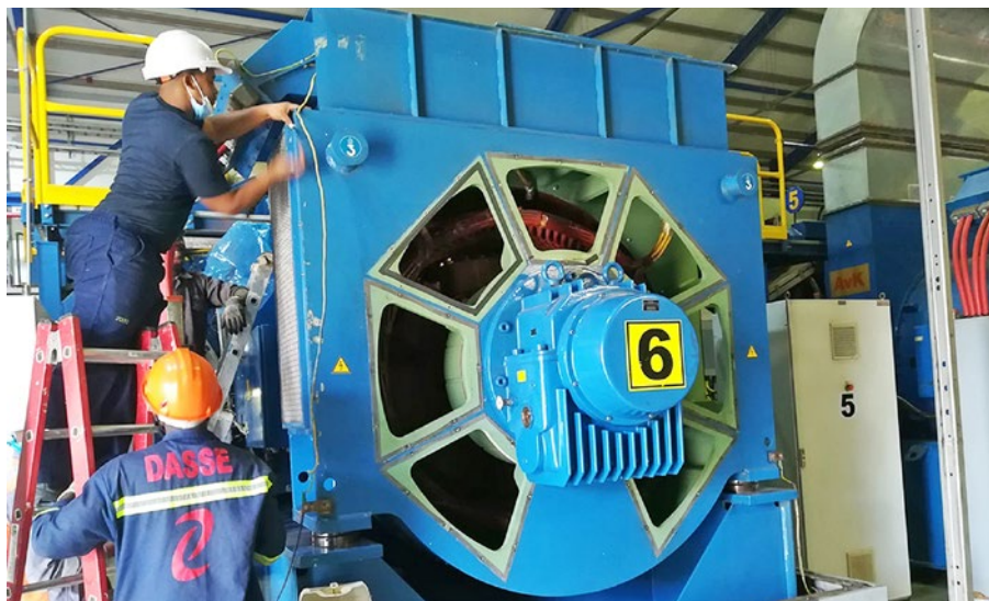
JP Cloete, a Field Service Technician of LHM's Rotating Machines division, is shown removing air filters from one of the six large alternators the field service team repaired on site at the diesel power plant serving Ndola in Zambia.
