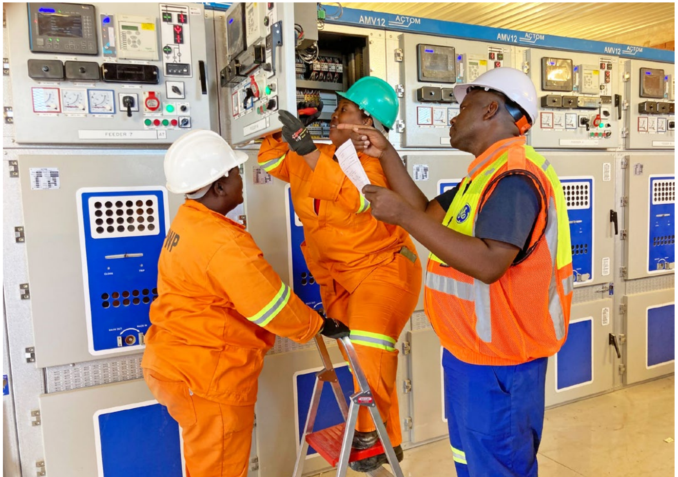
EPWP candidates assist with a wiring alteration on an AMV12 switchboard control cubicle under the watchful eye of Site Supervisor Kaizer Sithole at a substation in Tshwane that ACTOM Power Systems refurbished recently.
