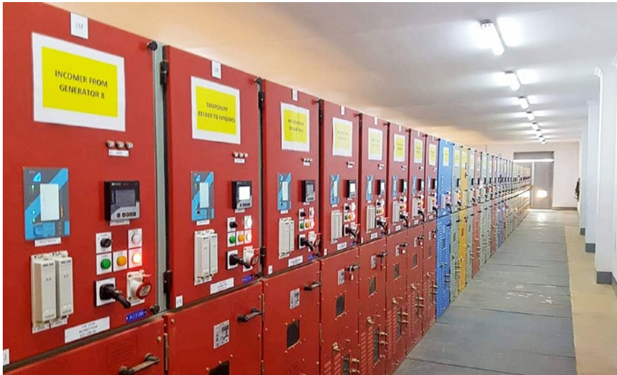
An array of switchgear panels in one of the eight surface substations at Kamoia mine that MV Switchgear has manufactured, supplied and installed the equipment for, with many more still due to be supplied for the mine's underground substations.
