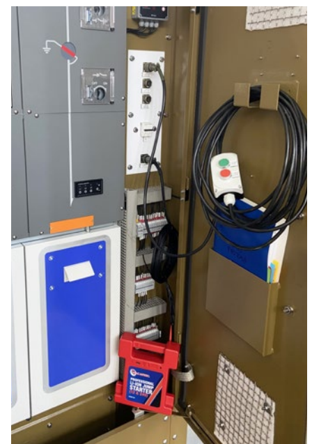
One of the RMV units supplied to Eskom KZN recently, complete with portable battery pack (bottom right) for remote operation.
